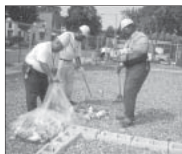
Friday, 10:15 a.m. — left to right: Steve Johnson, substation technician, Elton Pittman, construction maintenance first class, and Aaron Tyler, gardener class A.
